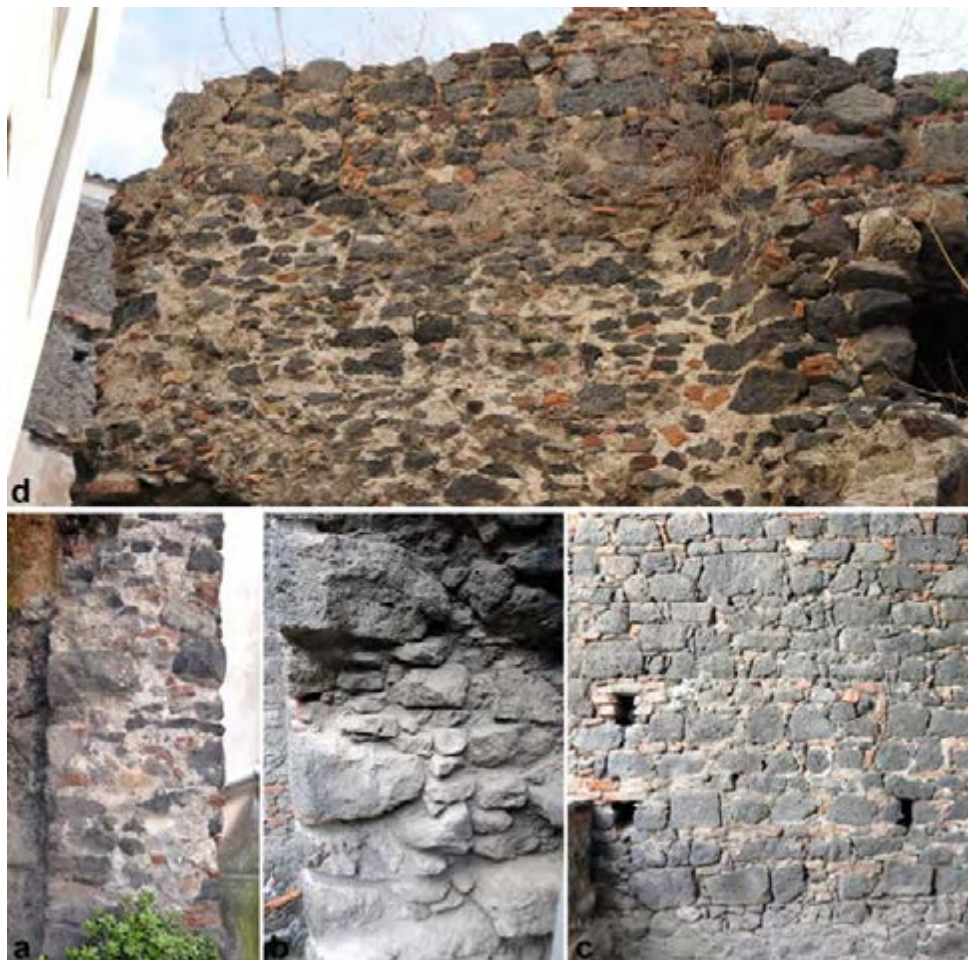
Fig. 12. Wall section in room 2 (a) and 11 (b); crusta in room 1 (c); detail of the fartura in the western wall of room 2, where the crusta is missing (d).
