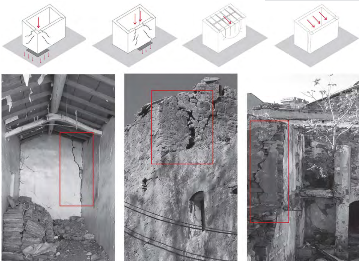
Figure 4. Recurring forms of degradation of masonries.
