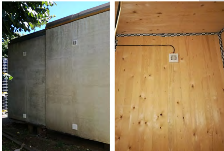
Figure 9. North façade of the test box. The white elements on the façade represent the ventilation extract fans and the ventilation grilles. The Test 3 was set to analyze the night ventilation effect on the two analyzed envelope technologies.
