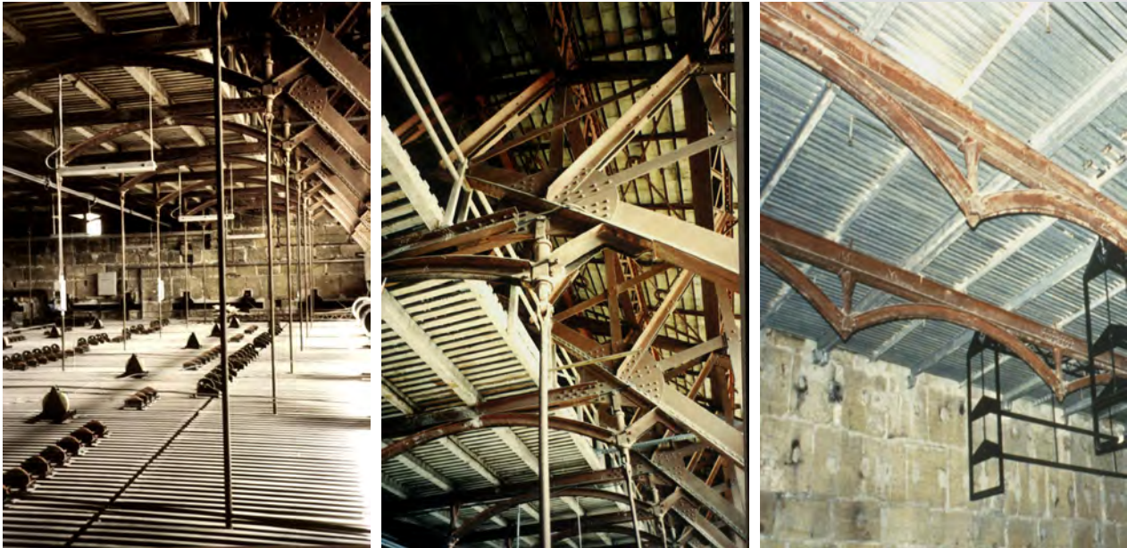
Figure 4. Teatro Massimo: the metal structure supporting the “cieli forati”, hanged up to the great arches of the stage roofing.
