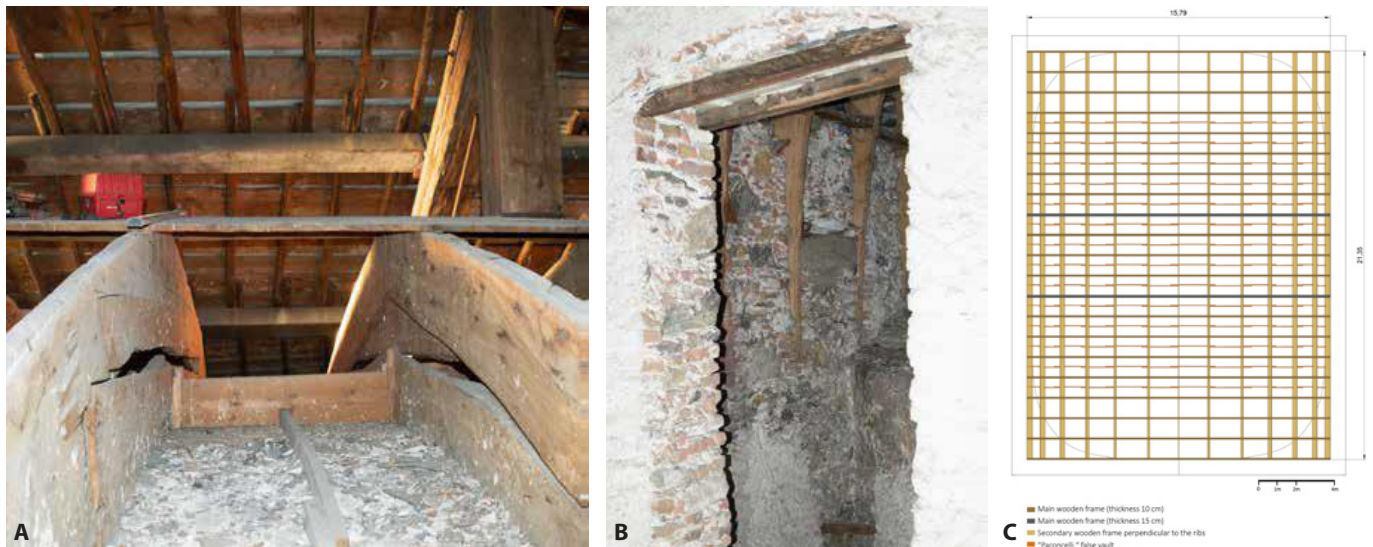
Fig. 4. A - Detail of the curved profile roof now devoid of the roofing mantle and protected by the gable roof. In the foreground, the reed vault of the inverted keel vault can be seen. B - Detail of the lower part of the ribs of the curved roof. C - Diagram of the curved roof structure (Image source: Accomasso 2019).
