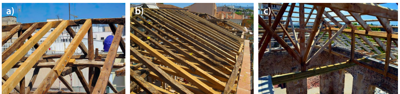
Fig. 9. New timber beams used to replace only the severely damaged rafters (a, b) [18]. The Neoclassical School in the Medieval city of Rhodes: New timber glued laminated beam replaced the poorly constructed original horizontal beam (c).
