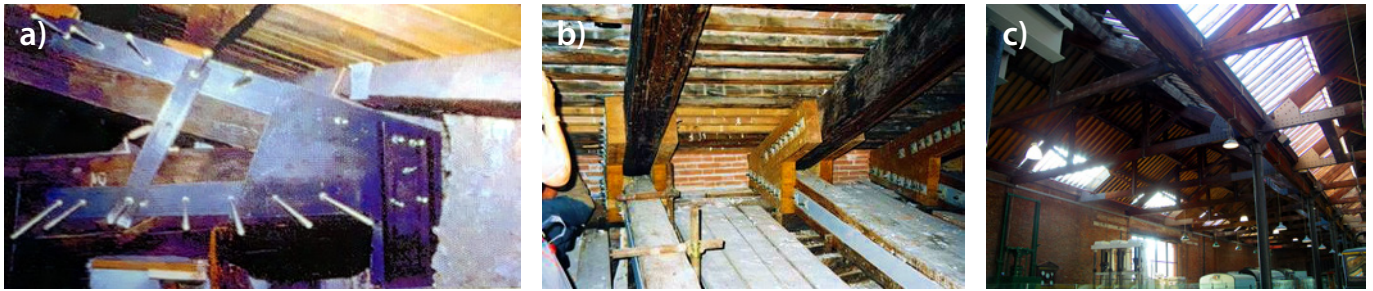
Fig. 11. Interventions that may change the stiffness properties of the original semi-rigid joints [20].
