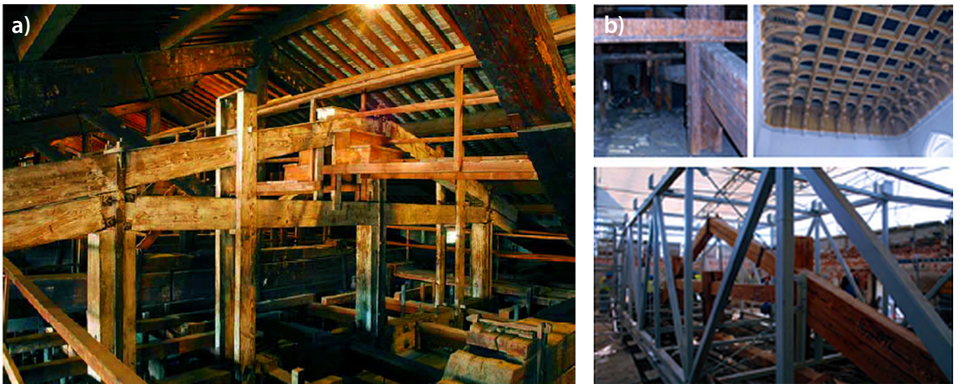
Fig. 13. Salone dei Cinquecento in Palazzo Vecchio, Florence. General view of the two trusses for the roof at the back of the photo (the original one) and the new one at the front (a) [25]. Main Railway Station in Wroclaw: A new load-bearing structure for the ceiling (a steel space frame) was used to relieve the roof truss from the coffer ceiling loads (b) [26].
