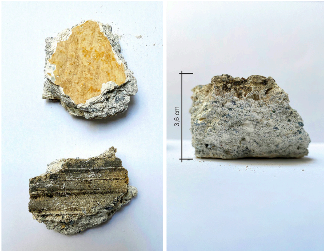
Fig. 8. Detailed photo of a portion of plaster of the timber structure vault.
