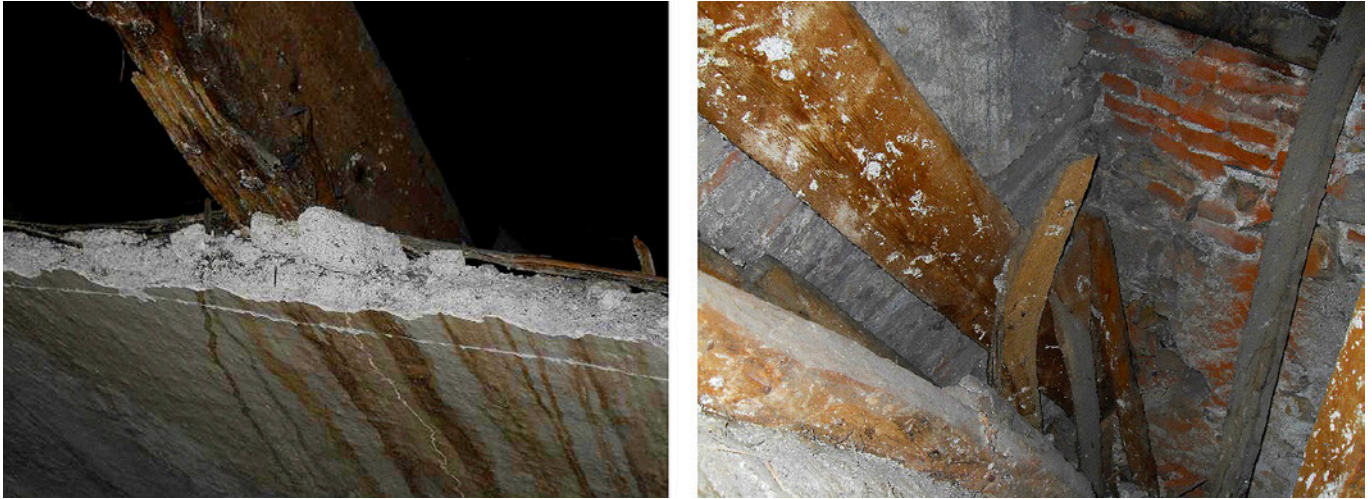
Fig. 10. The collapsed area of the vault and masonry wattle and disjoining in the support area of the struts.
