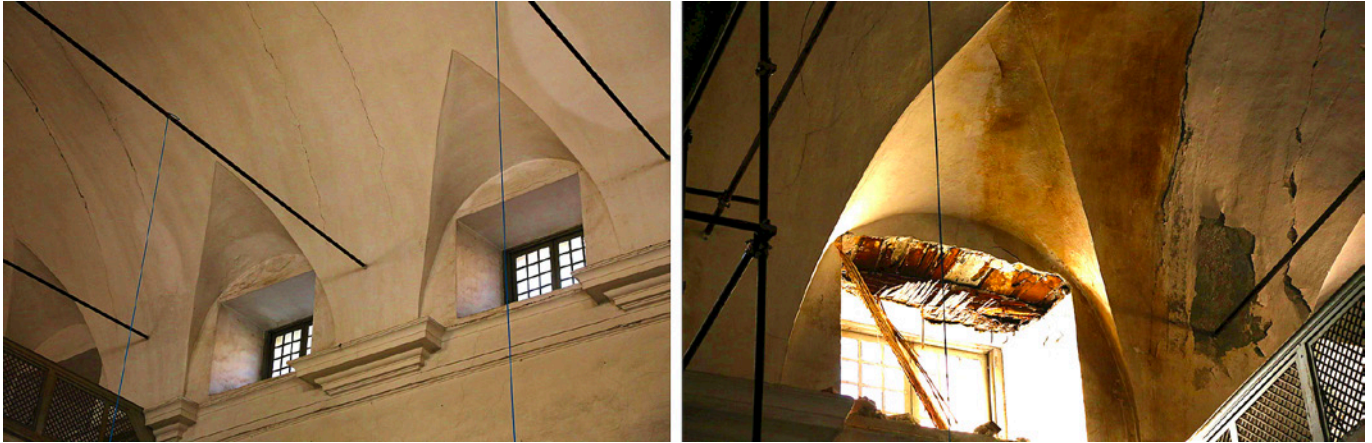
Fig. 6. Longitudinal cracks in correspondence of the arches and partial lack of the wattle of the ceiling above a window on the south side.
