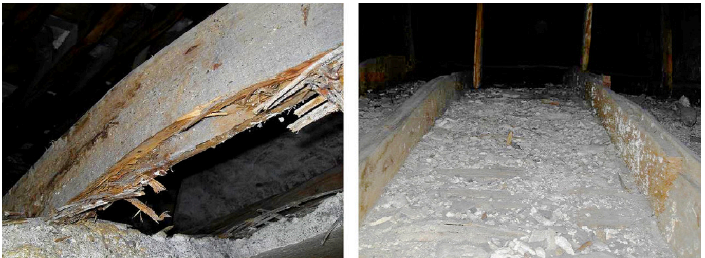
Fig. 11. Degradation of the ribs and presence of loose material on the vault.
