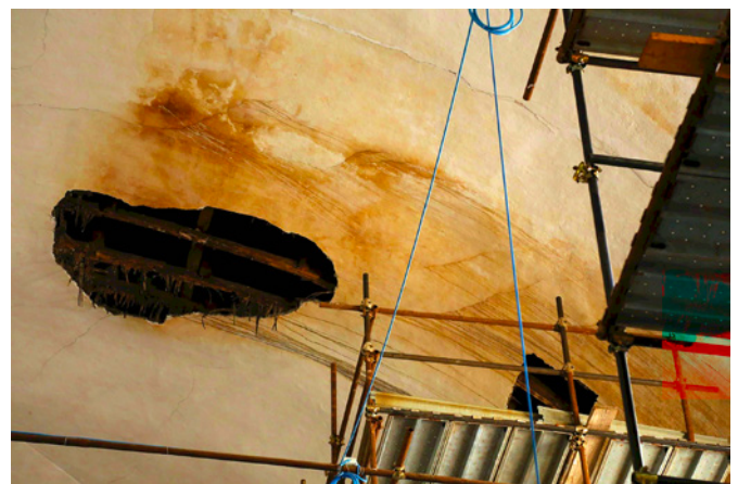
Fig. 7. Detail of the vault with the collapsed portion of wattle and plaster.
