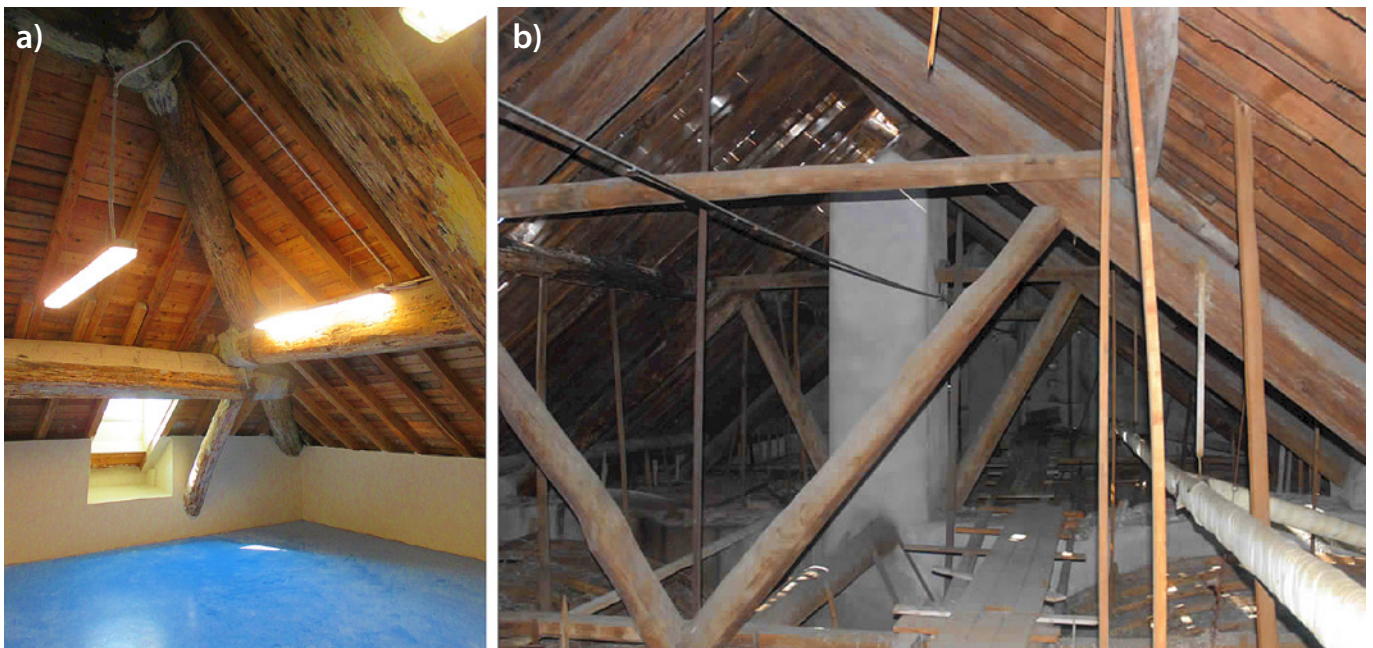
Fig. 1. Examples of the two types of roof structures present in the Albergo dei Poveri complex: (a) the roof structure of the west tower in the south wing of the complex; (b) the roof structure of the west side of the north wing.
