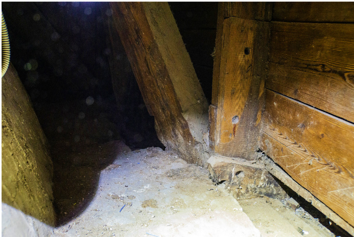
Fig. 7. Relics dome: cover plates supported by short wooden blocks to follow the projecting profile of the outer shell.
