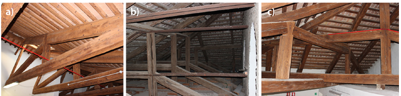
Fig. 5. Timber roofs types: (a) asymmetrical king trusses; (b) asymmetrical queen trusses reinforced with fitch plates at the joints and a double layer of tie rods; (c) intersection between asymmetrical queen trusses.
