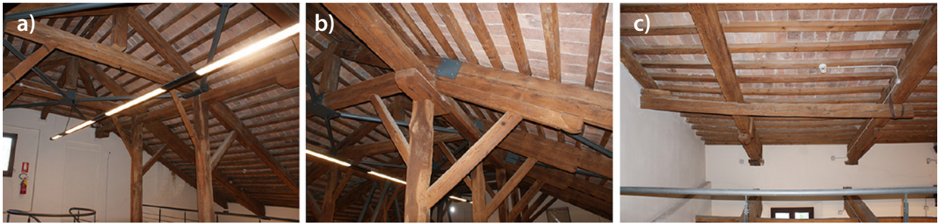
Fig. 6. (a) Timber rafter roof with crown posts; (b) connection between collar purlins highlighted by the presence of a wooden capital; (c) previous reinforcement for excessive deformation.
