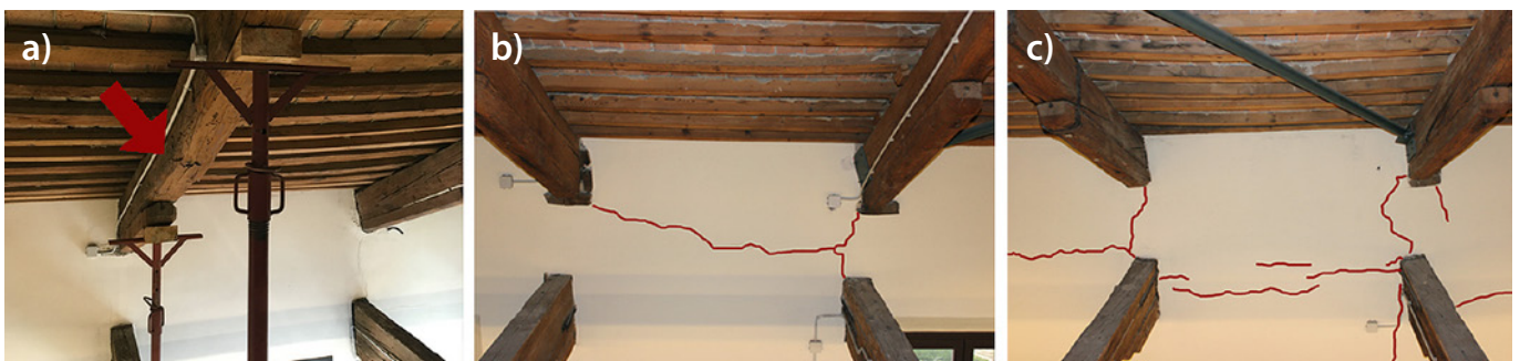
Fig. 7. Seismic damages: (a) cracked rafter; (b, c) horizontal masonry cracks on longitudinal walls.
