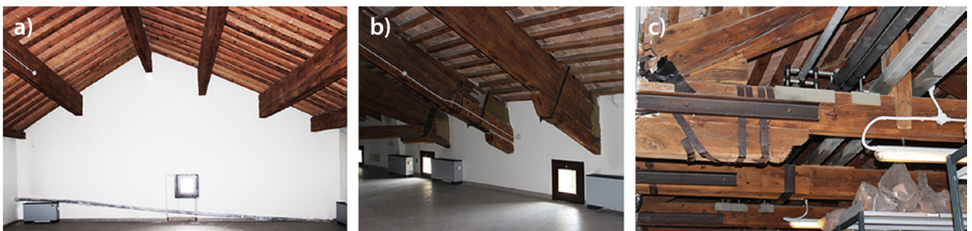
Fig. 4. Timber roofs types: (a) large-span timber purlin roof built with the "trave composta" technique; (b) timber rafters roof made with the "trave composta" technique; (c) a small-span king trusses roof with reinforcement.
