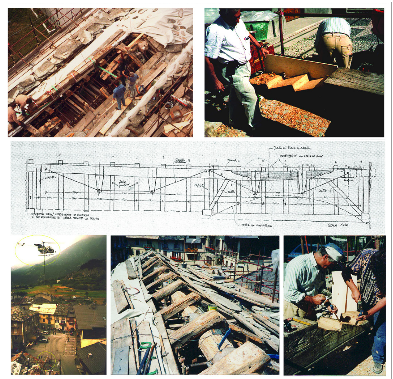
Fig. 10. Phases of the interventions carried out in 2000 with the integration of timber elements, the realization of the double "dart of Jupiter" joint, the transportation of the larch beam on the construction site, some details of the steel elements of the reinforced beam, and the scheme of the reinforcement intervention with Polonceau system. (Image source: drawings and photos courtesy of C. Bertolini-Cestari).
