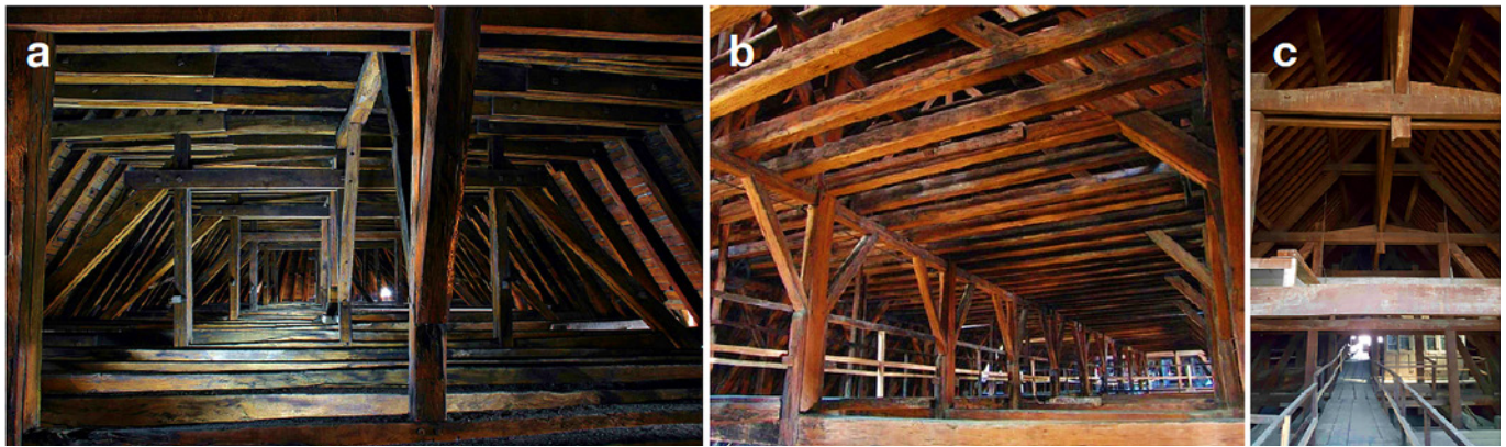
Fig. 2. Views of the combles: (a) in the choir (image source: [7]); (b) in the nave (image source: [8]); (c) in the transept (photo by the Author).
