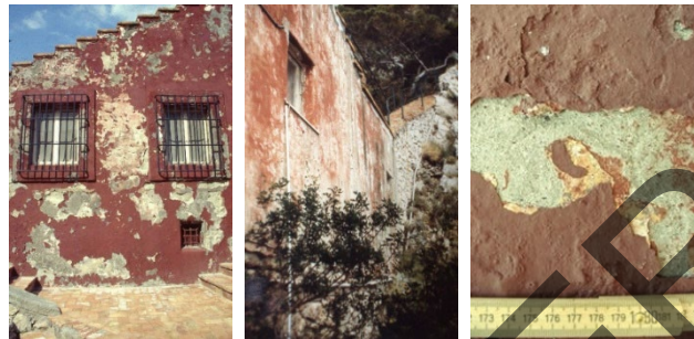
Fig. 02a,b,c: A. Libera, Malaparte house, details. The state of degradation of the paintwork and the complex layering can be seen (source: Pertot archive).
