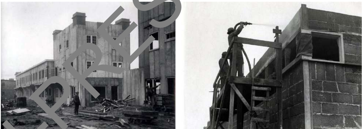
102 103 104 Figure 4 Quartiere Betondorp (1921-30) view of the construction site of a building made with «B.B.B. - Bims Beton 105 Bouw» (left) e «Hunkemüller» (right)
