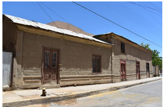
Fig. 9. Decorated façade of Pisco Elqui, Elqui Valley. Source: picture by Elena De Santis, 2022.
