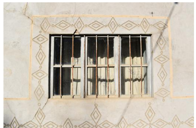
Fig. 5. Decorated façade of Tulahuén, Limarí Valley. Source: picture by Elena De Santis, 2022.
