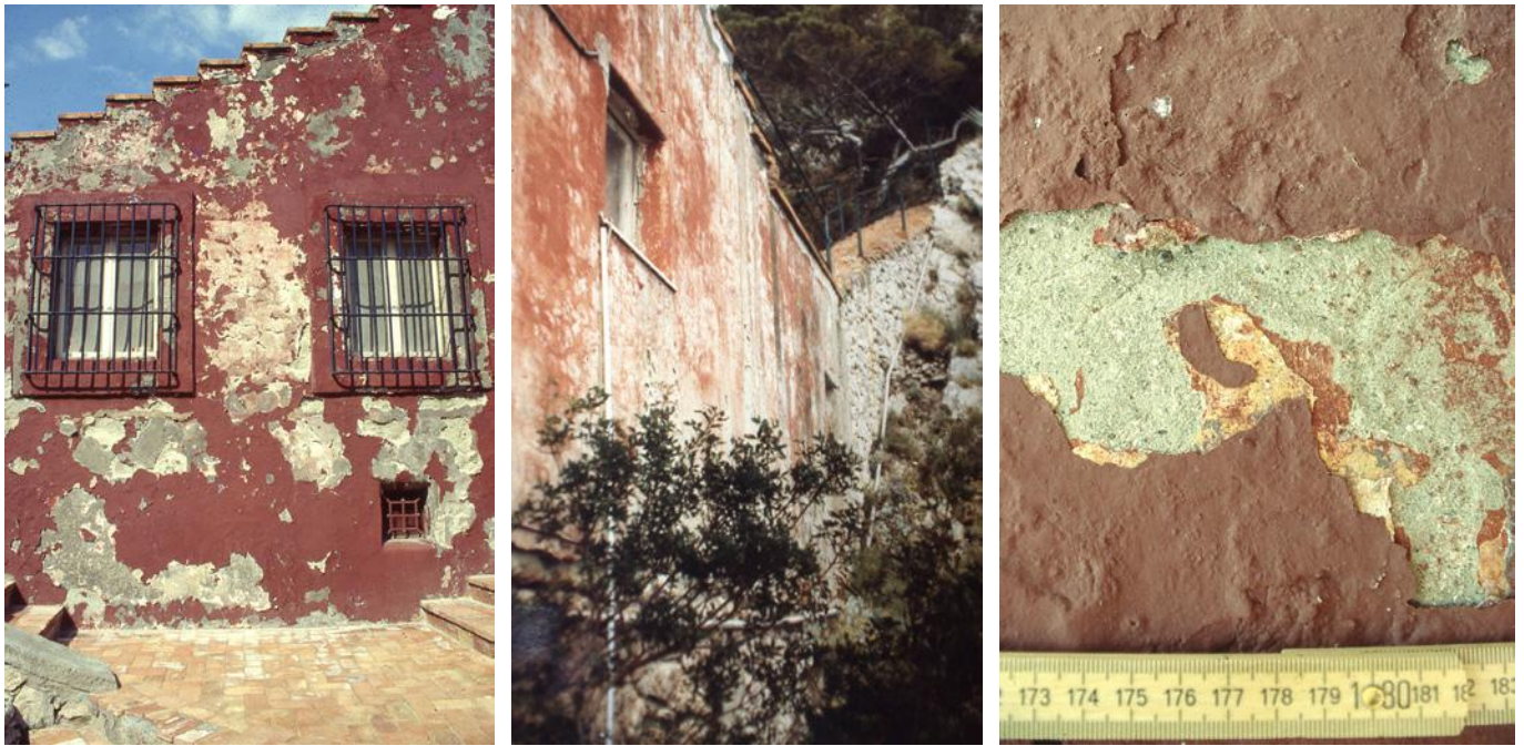
Fig. 2. A. Libera, Malaparte house, details (left, center, right). The state of degradation of the paintwork and the complex layering can be seen. Source: Pertot archive.
