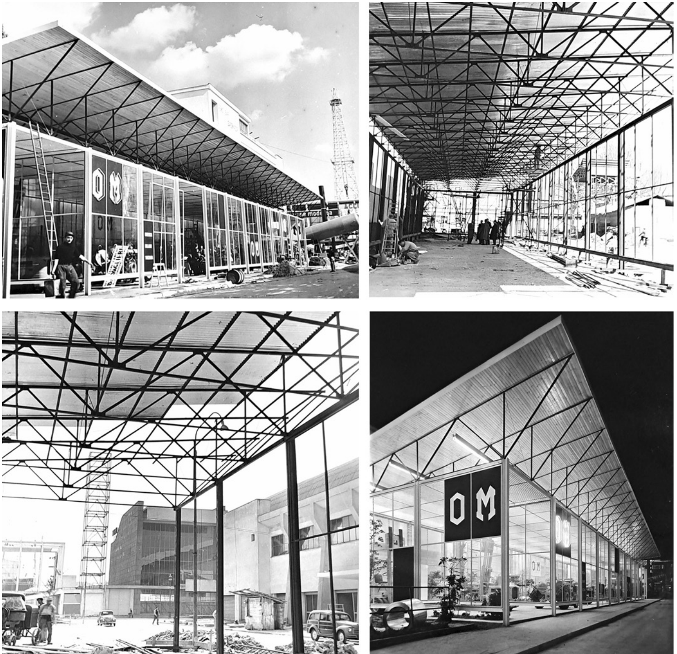
Fig. 4. The OM pavilion of 1953 under construction. Source: CSAC, Università di Parma, Renzo Zanavella Collection.
