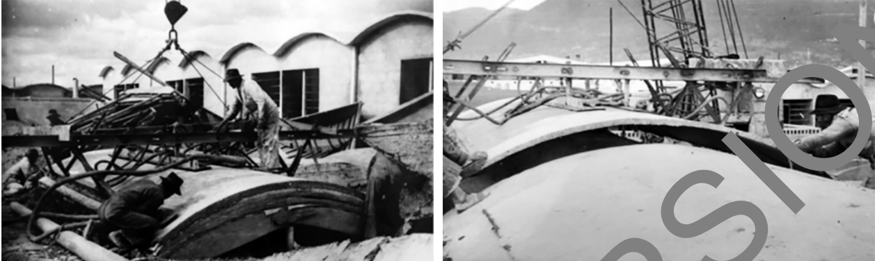
295 296 Fig. 6. Left: Construction of the shells above a wooden formwork with vacuum concrete. Right: Setting a shell as a roofing for a 297 residential unit through the Vacuum Lifter method. Images by Galindo-Diaz et al., 2022.
